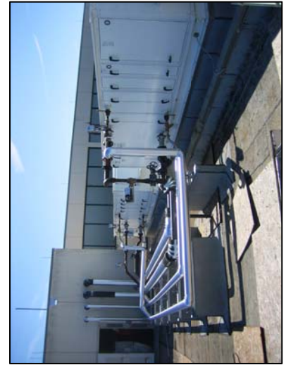
Roof top Equipment Piping
